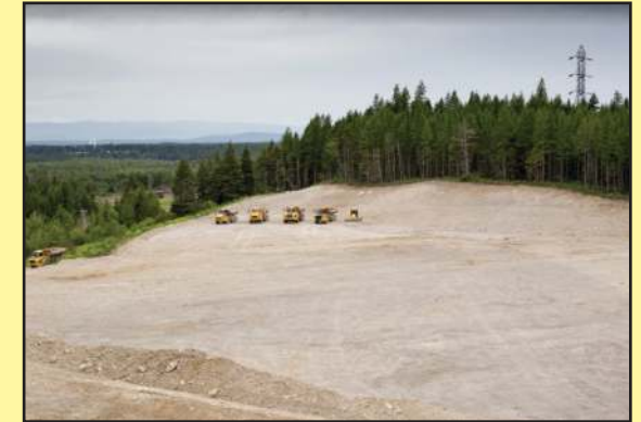
On-site gravel pit where backfill materials are obtained to fill potroom basements.
